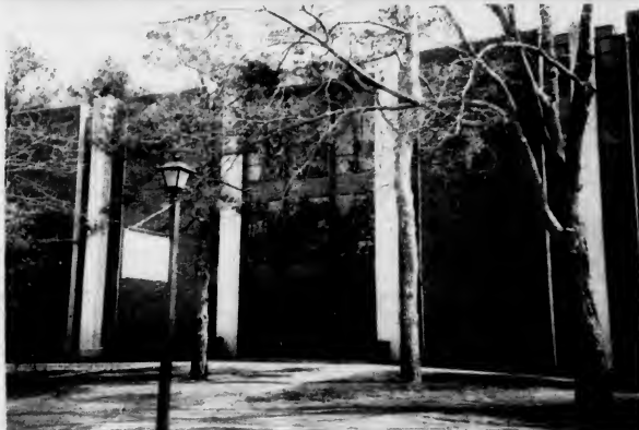
Renovations to the basement of Hawthorne-Longfellow Library have begun after seven years of planning. (Sherri Kies/Bowdoin Orient)
